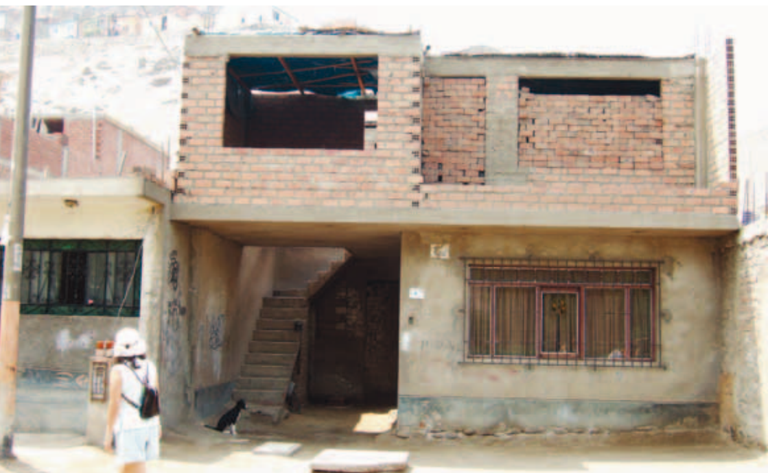
Rental units under construction in informal settlements in the periphery of Lima, Peru.
